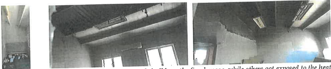
Extent of damage varies, as some rooms were sealed off from the fire damage, while others got exposed to the heat and smoke
