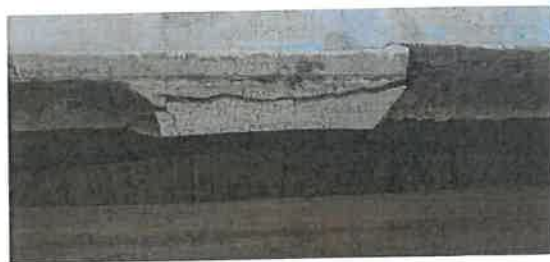
Plaster hanging on concrete beam - H&S risk
