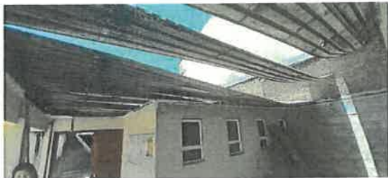
Roof sheets with nails through is a safety risk
