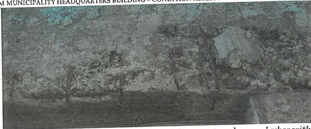
Photo 3.8: Internal concrete beam, with spalling of the concrete and exposed rebar with visible corrosion. The concrete cover on these concrete beams seems to have deteriorated, due to the heat of the fire damage.
