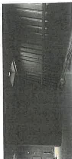
Passage way with severe smoke damage
