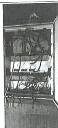
DB made safe by client
