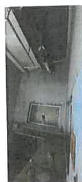
Reception area with smoke damage at the roof.
