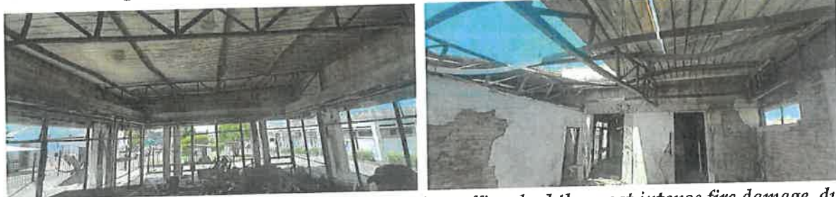
Photo 3.1 & 3.2: Geodebt offices and Financial services offices had the most intense fire damage, due to many documents stored in the building that fuelled the fire. Large open windows allowed some of the heat to escape out of the building and that is why the roof structure did not collapse, even though the fire was very intense.
