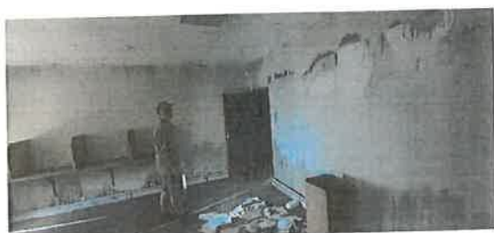
Room with smoke damage
