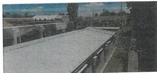
Back building roof and damaged roof visible
