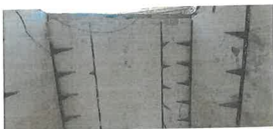
Records room where the walls are severely cracked
