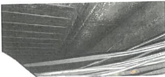
Ceiling void smoke damage
