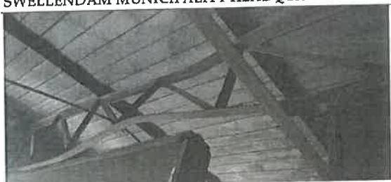
Bent truss from heat of fire
