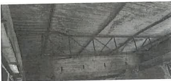
Steel truss with localized buckling of some members
