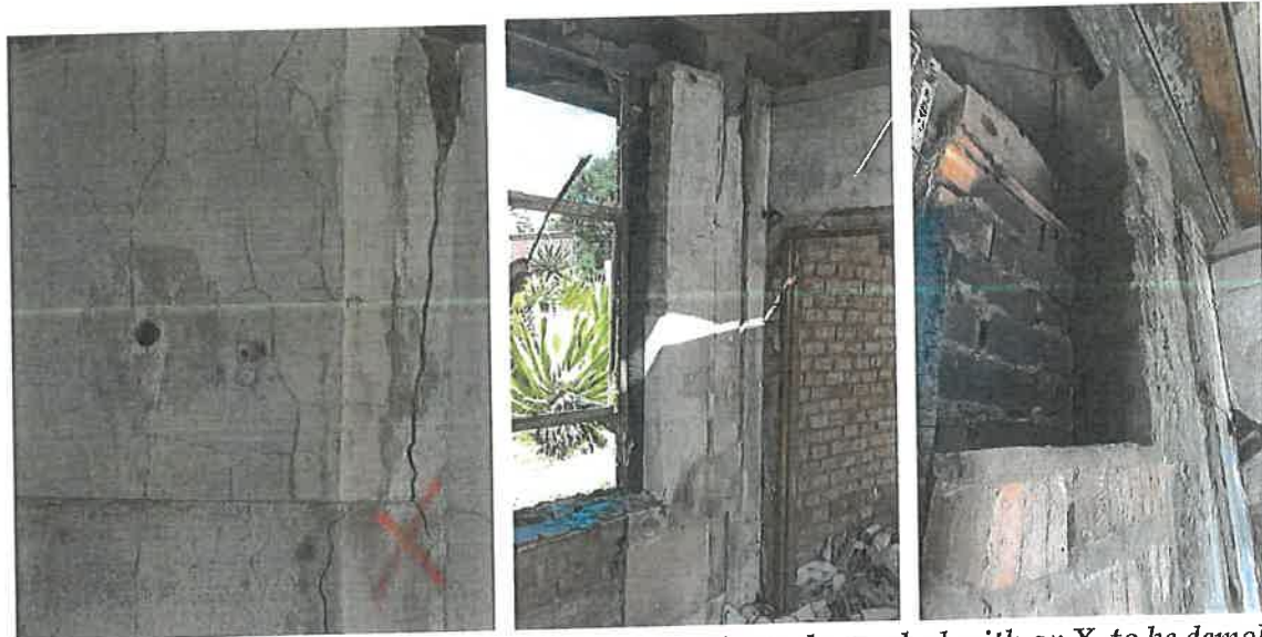
Photo 3.3: Example of typical brick wall with large visible cracks marked with an X, to be demolished. Photo 3.4 & 3.5: Brick wall nibs around timber window frames have lots of heat damage in the cavities that are not so obvious, from a visual assessment only.
