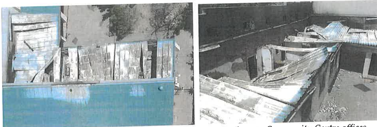
Photo 2.2& 2.3: Close up view of the fire damage to the Thusong Community Centre offices
