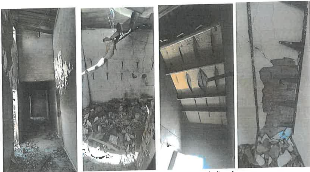
Photo 3.4 Passageway with high roof with fire damage.
