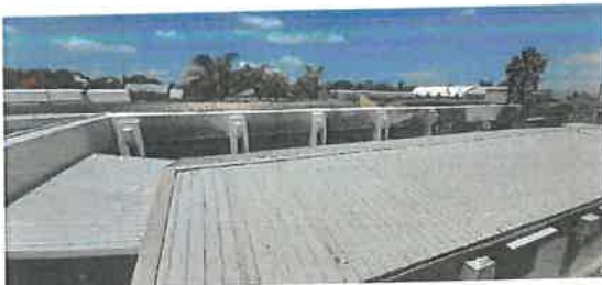
Back view with smoke damage visible
