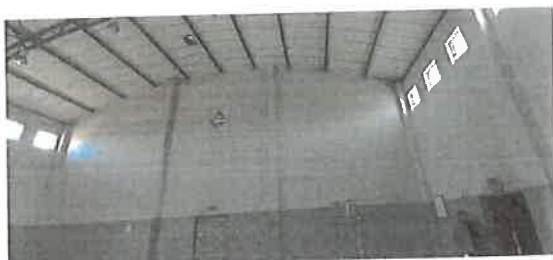
View of hall eaves with slight smoke damage in top right corner.
