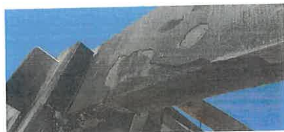
Concrete frame with spalling plaster
