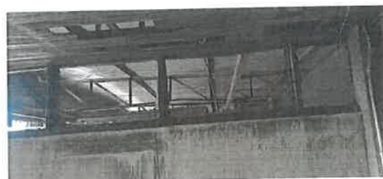
Roof structure visible due to damaged ceilings
