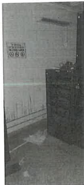
Server room rated 3
