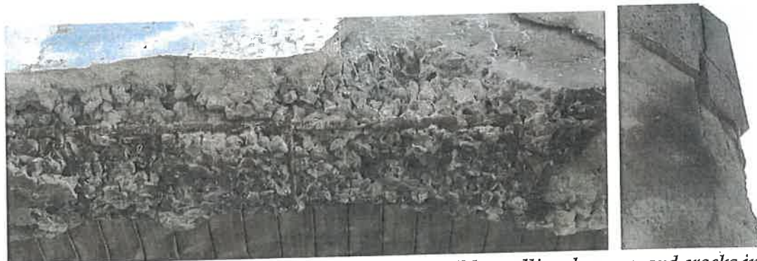
Photo 3.6 & 3.7: Concrete beam on façade with localized visible spalling damage, and cracks in concrete façade beam. Note the visible corrosion that is related to the heat damage that will also start forming at the rest of the rebar in the heat-damaged concrete, where oxygen can reach the rebar.
