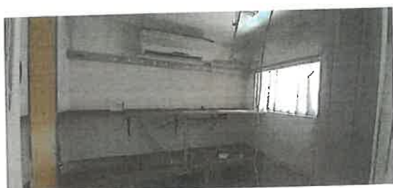
Old server room rated 4
