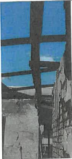
Truss bowing due to fire damage
