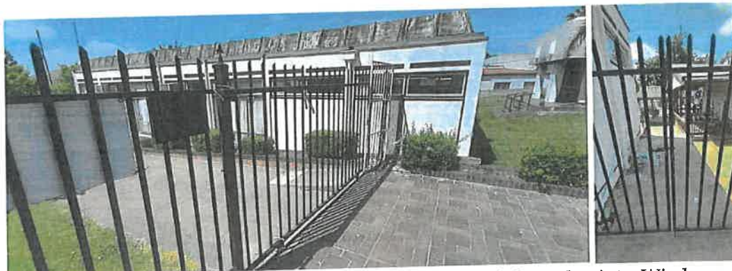
Photo 3.11 & 3.12: Sliding gates on the perimeter fence is damaged, from the riots. Windows were also damaged on the adjacent buildings, during the riots.
