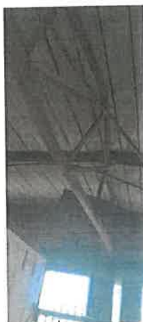
Records room with bent steelwork rated 1
