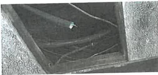
Ceiling void hall 2 smoke damage
