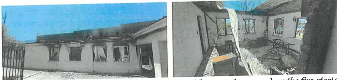
Photo 3.1 & 3.2 Thusong community centre offices with severe damage where the fire started.
