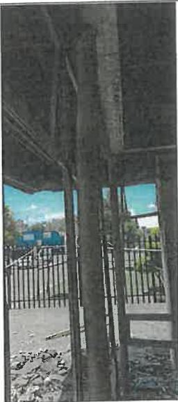
Steel post bent due to fire damage
