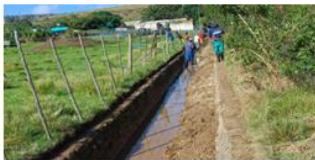
Cleaning and Maintenance Program
