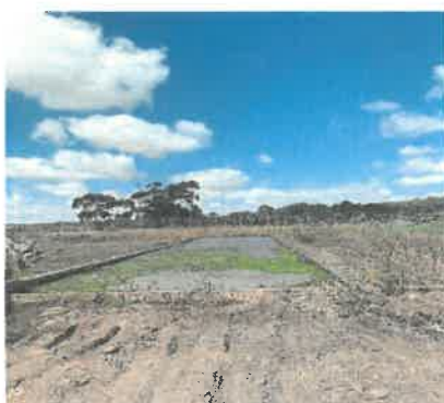
Poorly Maintained Sludge Drying Beds
