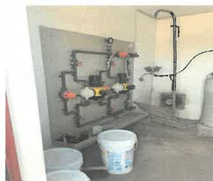
Chlorine Room Not Equipped with CCTV Cameras
