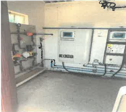
Unauthorized Access in the Chlorine Room
