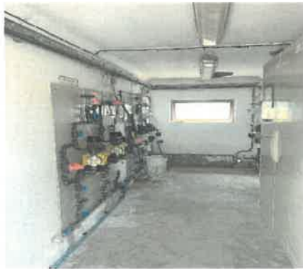
No CCTV Cameras in Chlorine Room
