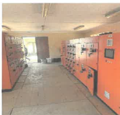
No CCTV Cameras in the Electrical Room
