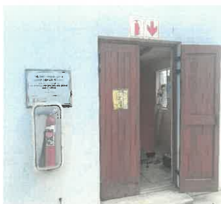
Unauthorised Access in the Electrical Room
