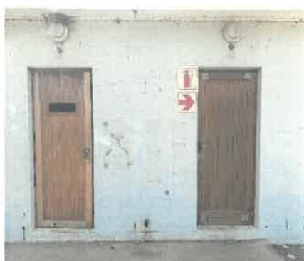
No Safety and Hazards signs in Chlorine Room
