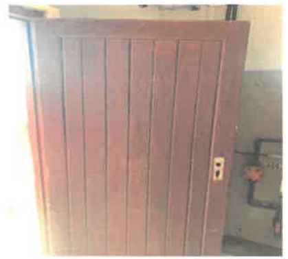
No Safety and Hazards Signs/Warnings in Chlorine Room
