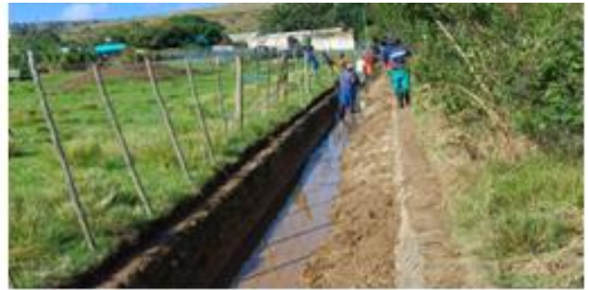
Cleaning and Maintenance Program
