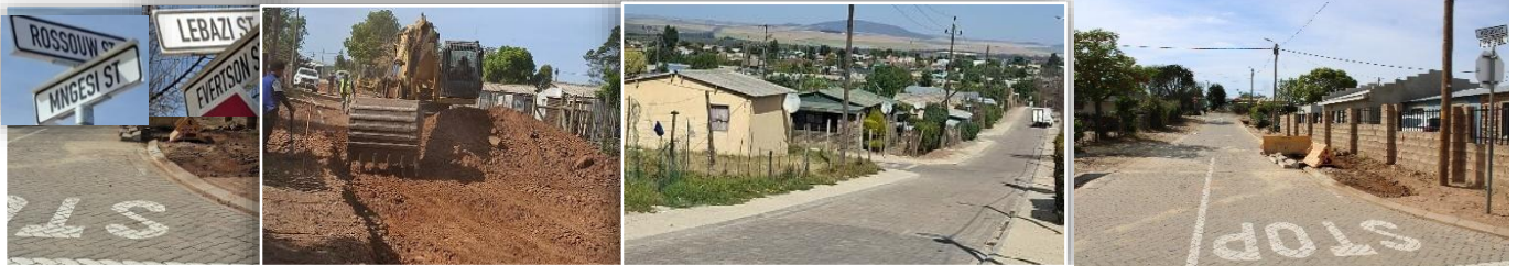
Railton Rising Main
